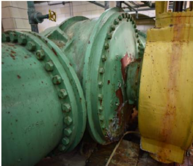
A 36-inch Cone Valve of GLWA
